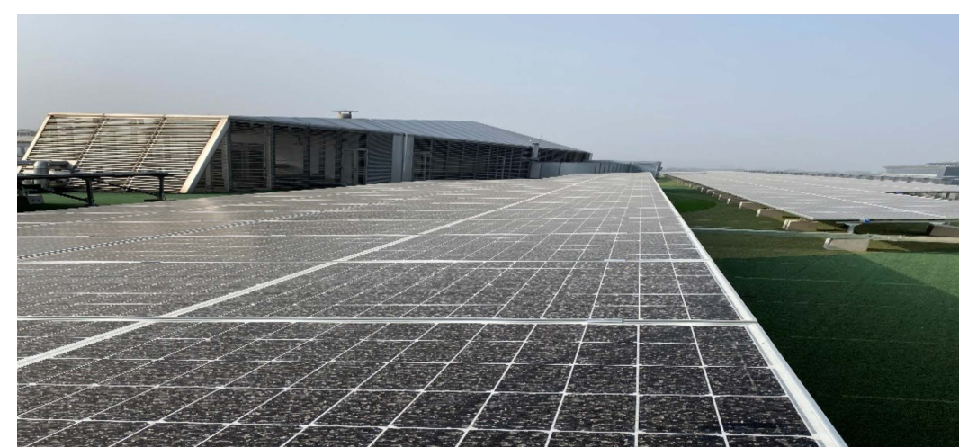
Distributed photovoltaic equipment on the roof
